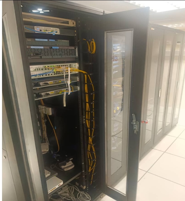
Existing Customer Equipment Rack
