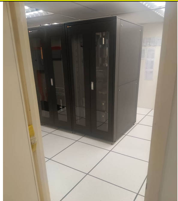
Existing Customer Server Room at Level 4, RHB Bank Building
