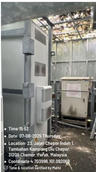
PICTURE 1 : CABINET UMOBILE
