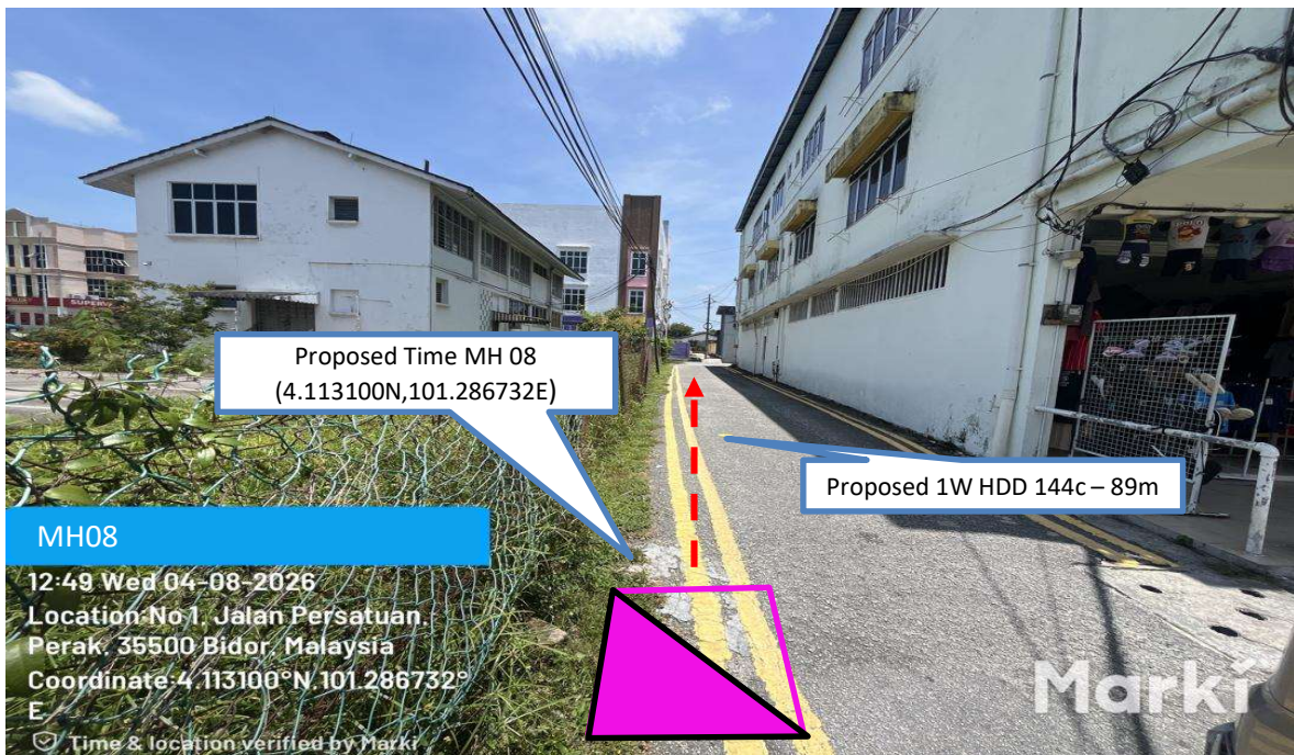
Prop 1W HDD 144C from Proposed Time MH08 n to Proposed Time MH09 - 89 m
