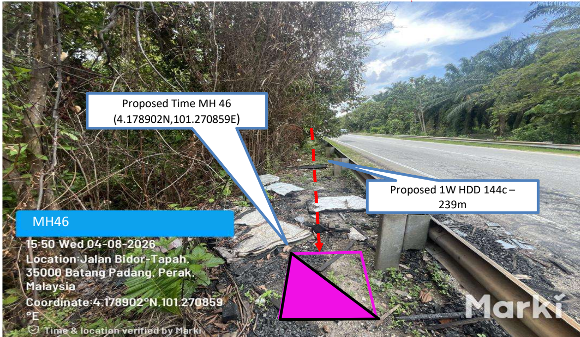
Prop 1W HDD 144C from Proposed Time MH45 n to Proposed Time MH46- 239 m
