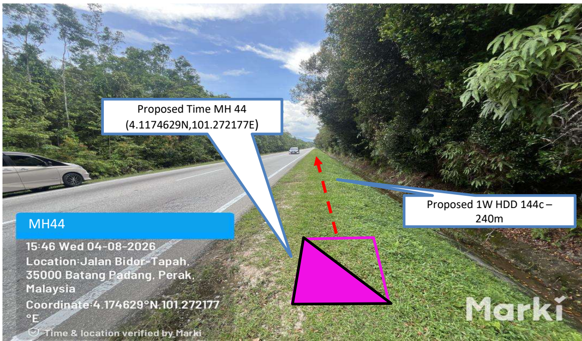
Prop 1W HDD 144C from Proposed Time MH44 n to Proposed Time MH45– 240 m
