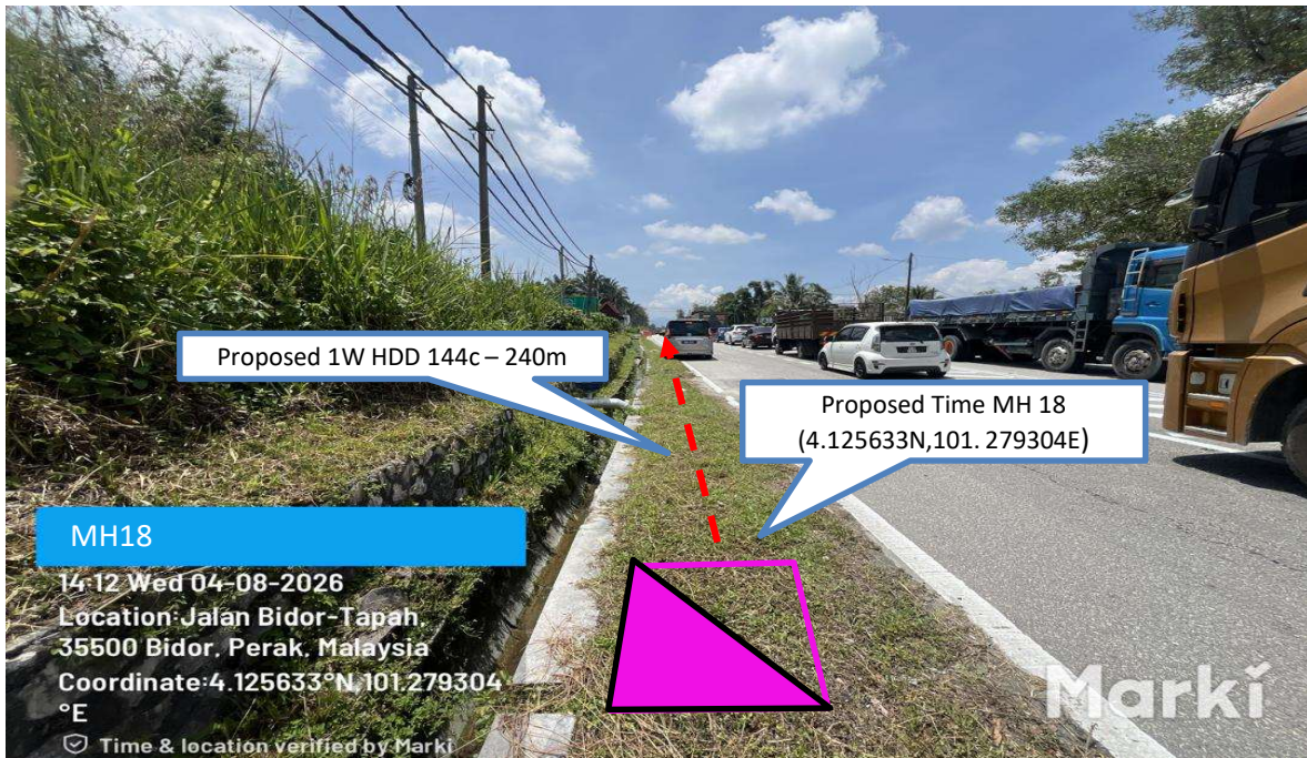
Prop 1W HDD 144C from Proposed Time MH18 n to Proposed Time MH19 – 240 m
