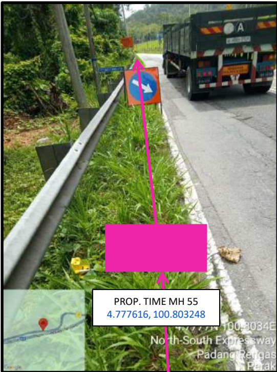
Proposed HDD 1 Way and Pulling Cable 144C from Prop. TIME MH55 to Prop. TIME MH56 at beside the highway
