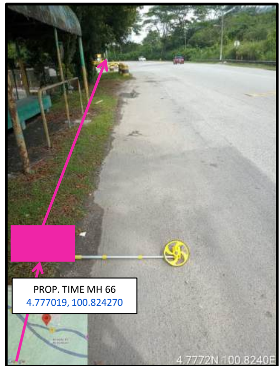
Proposed HDD 1 Way and Pulling Cable 144C from Prop. TIME MH66 to Prop. TIME MH67 at beside the highway
