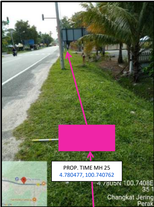
Proposed HDD 1 Way and Pulling Cable 144C from Prop. TIME MH25 to Prop. TIME MH26 at Jalan Enam Kaki
