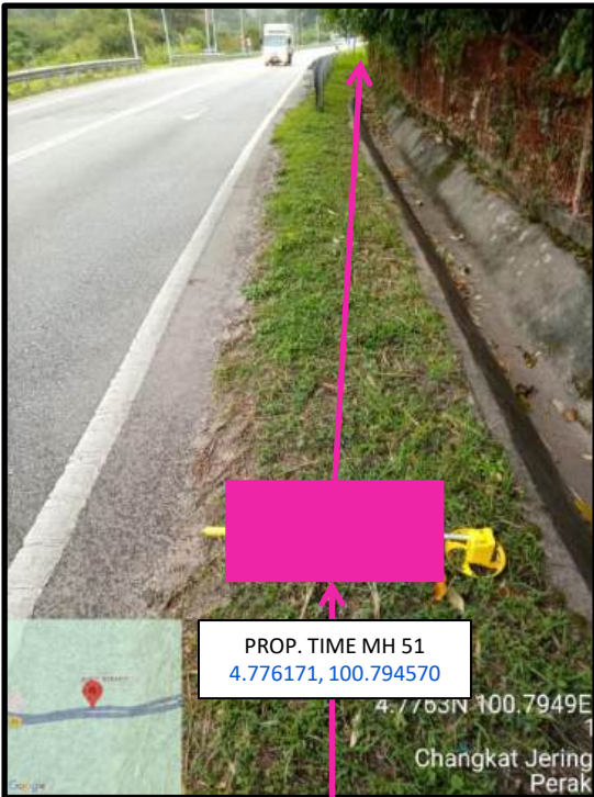
Proposed HDD 1 Way and Pulling Cable 144C from Prop. TIME MH51 to Prop. TIME MH52 at beside the highway
