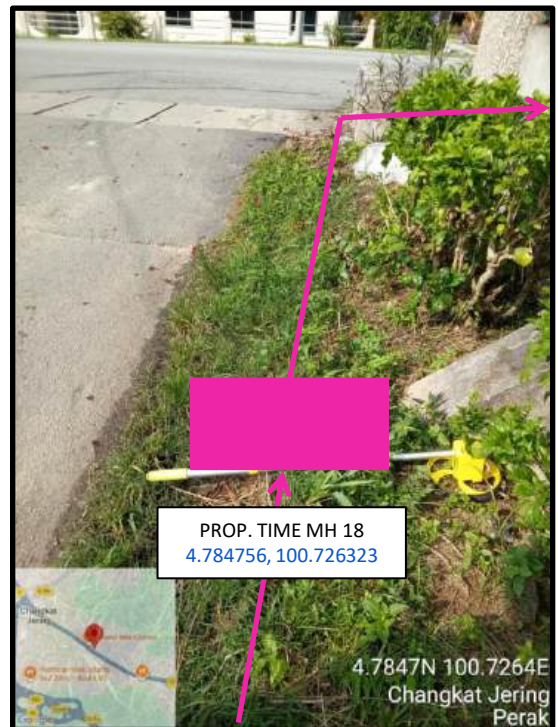
Proposed HDD 1 Way and Pulling Cable 144C from Prop. TIME MH18 to Prop. TIME MH19 at Jalan Enam Kaki
