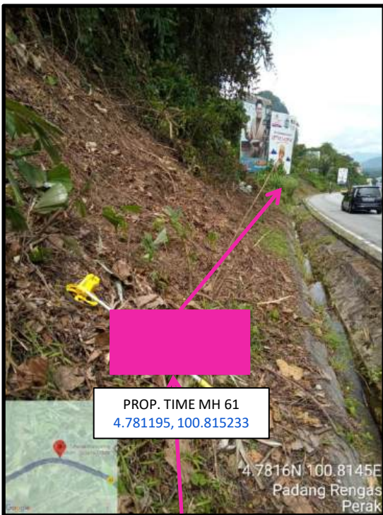
Proposed HDD 1 Way and Pulling Cable 144C from Prop. TIME MH61 to Prop. TIME MH62 at beside the highway
