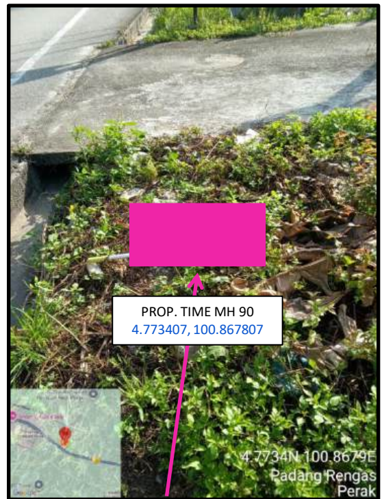
Proposed HDD 1 Way and Pulling Cable 144C from Prop. TIME MH89 to Prop. TIME MH90 at Padang Rengas
