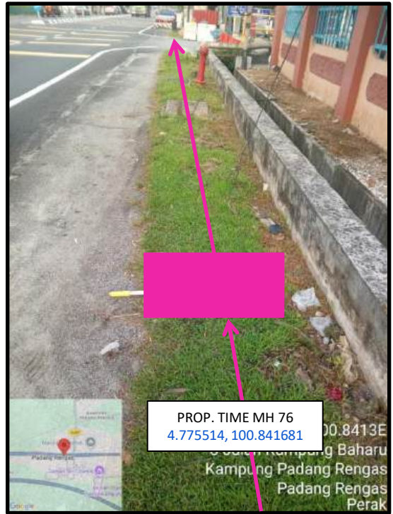
Proposed HDD 1 Way and Pulling Cable 144C from Prop. TIME MH76 to Prop. TIME MH77 at Kampung Baharu
