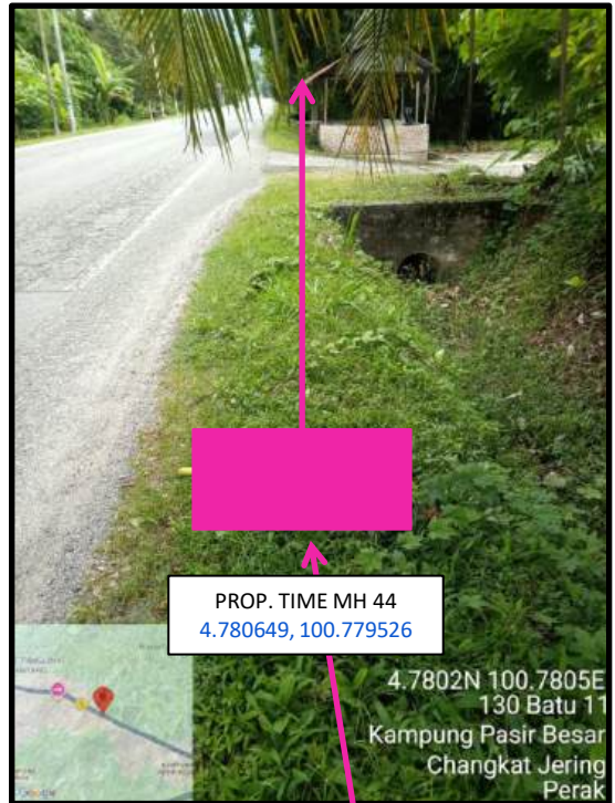
Proposed HDD 1 Way and Pulling Cable 144C from Prop. TIME MH44 to Prop. TIME MH46 at Kampong Pasir Besar
