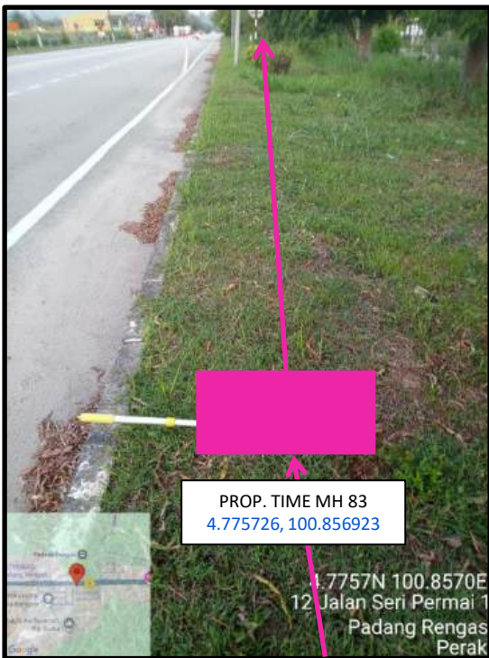
Proposed HDD 1 Way and Pulling Cable 144C from Prop. TIME MH83 to Prop. TIME MH84 at Jalan Seri Permai 1
