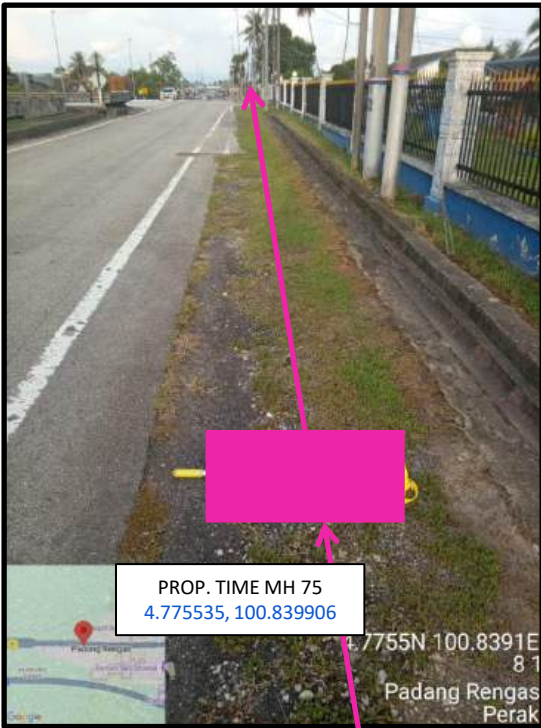
Proposed HDD 1 Way and Pulling Cable 144C from Prop. TIME MH75 to Prop. TIME MH76 at Kampung Baharu
