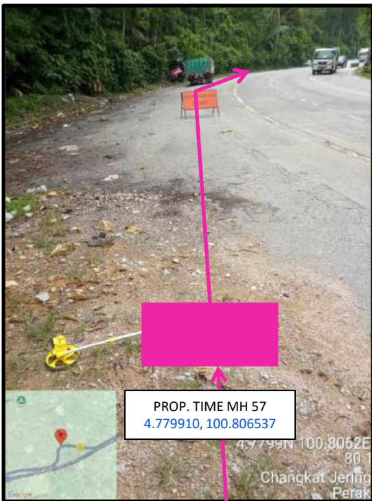
Proposed HDD 1 Way and Pulling Cable 144C from Prop. TIME MH57 to Prop. TIME MH58 at beside the highway
