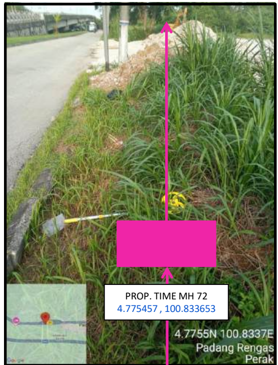
Proposed HDD 1 Way and Pulling Cable 144C from Prop. TIME MH72 to Prop. TIME MH73 at Kampung Padang Rengas
