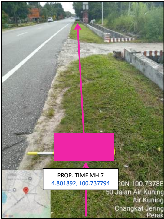
Proposed HDD 1 Way and Pulling Cable 144C from Prop. TIME MH07 to Prop. TIME MH08 at Jalan Air Kuning
