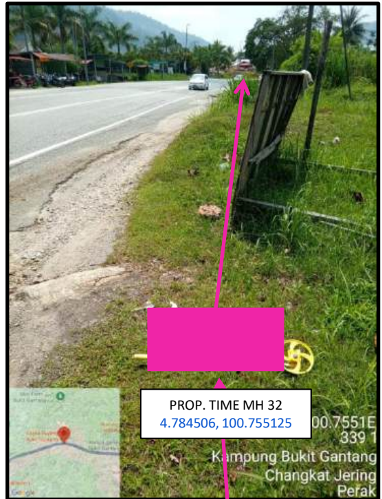
Proposed HDD 1 Way and Pulling Cable 144C from Prop. TIME MH32 to Prop. TIME MH33 at Kampong Bukit Gantang
