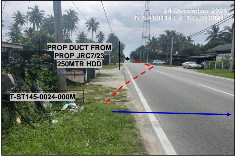
LOCATION AT JALAN (T145)
