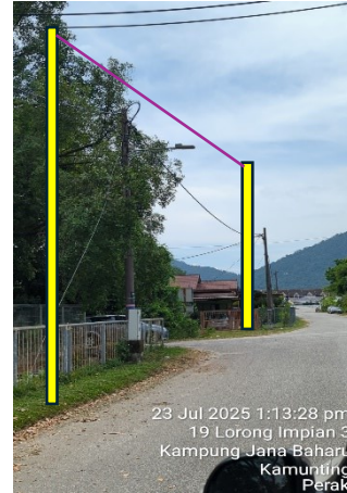
PROP POLE AT LORONG IMPIAN 3
