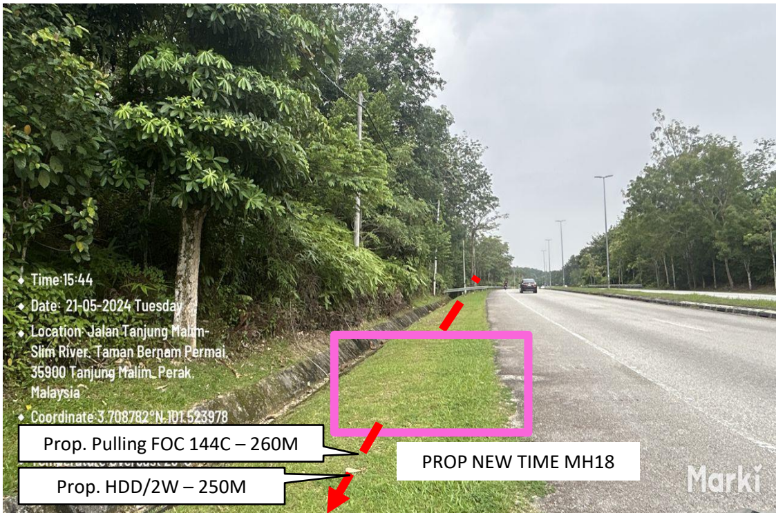
Proposed HDD/2W (250M) and pulling FOC 144C (260M) from Prop New TIME MH18 to Prop New TIME MH19
