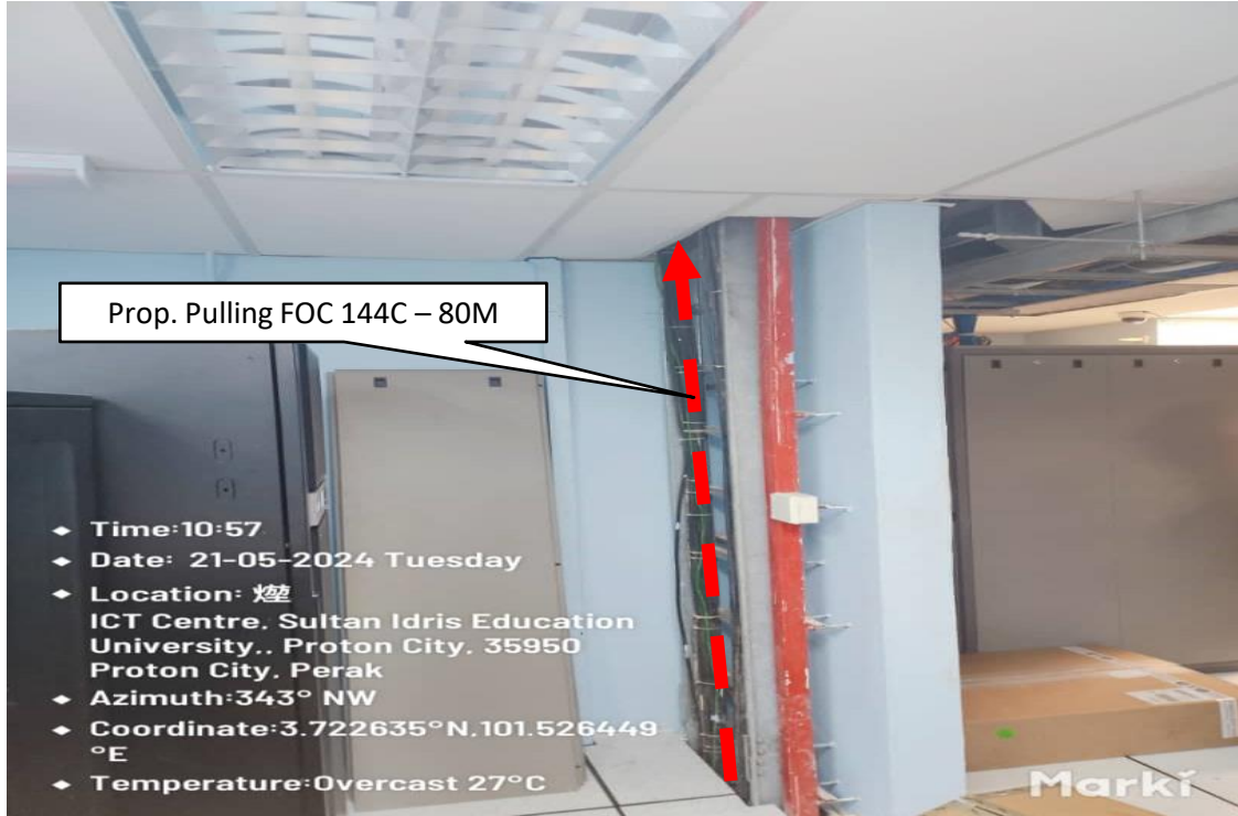
Proposed Route for new Cable 144C from Server Room at Level G, Pusat ICT using existing cable tray – 80m.
