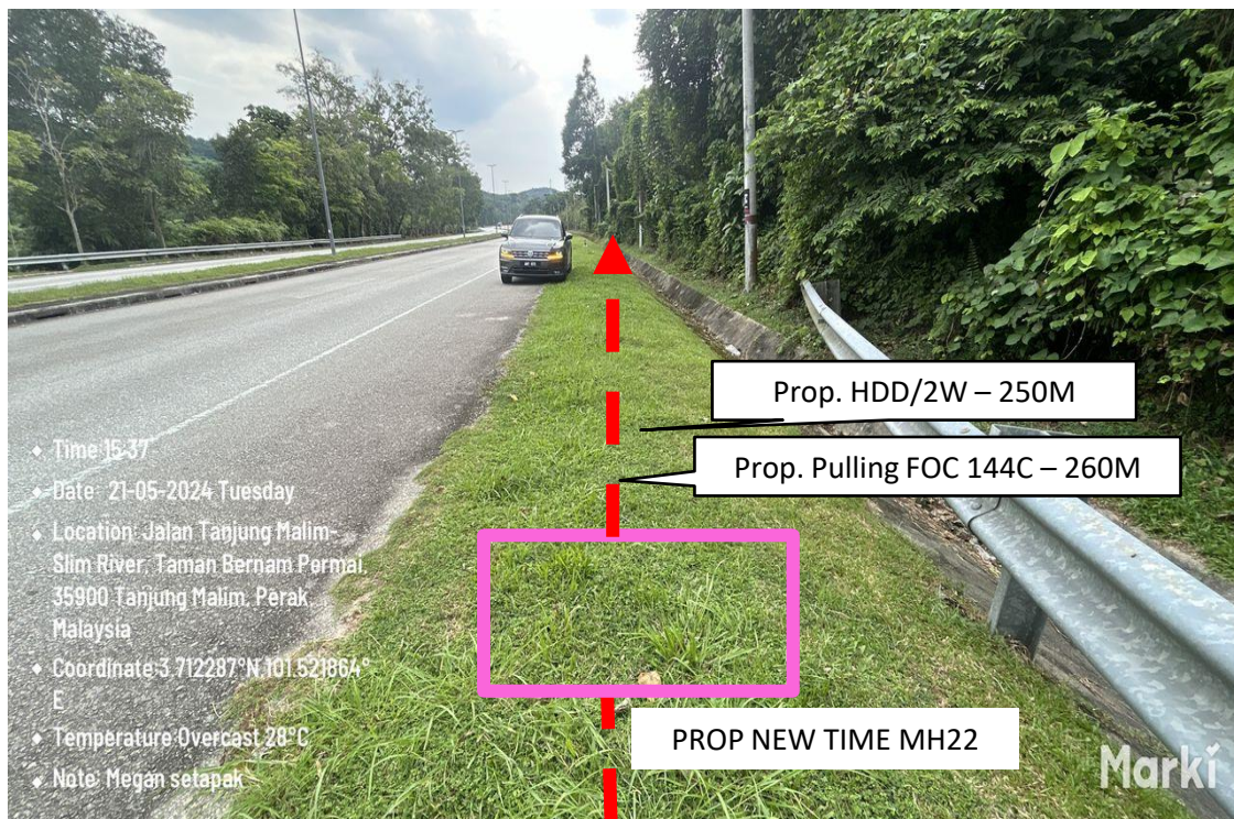
Proposed HDD/2W (250M) and pulling FOC 144C (260M) from Prop New TIME MH22 to Prop New TIME MH23
