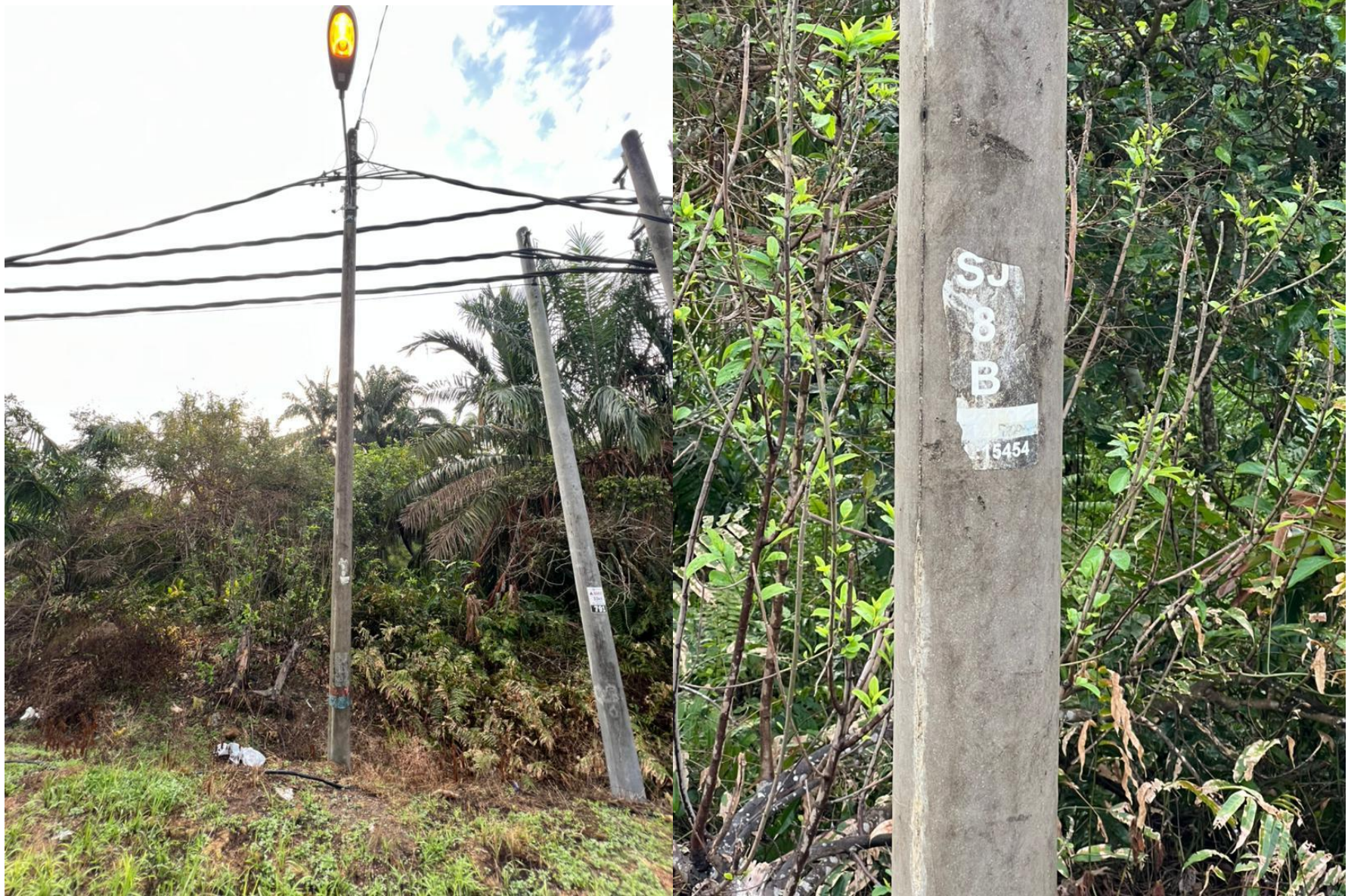
TNB Pole 5.1855565596689, 100.6761967119 *HDD starting point
