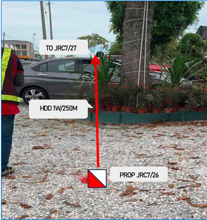
PROP JRC7/26 LOC AT JALAN TAMBUN BARU (ROADSIDE)
