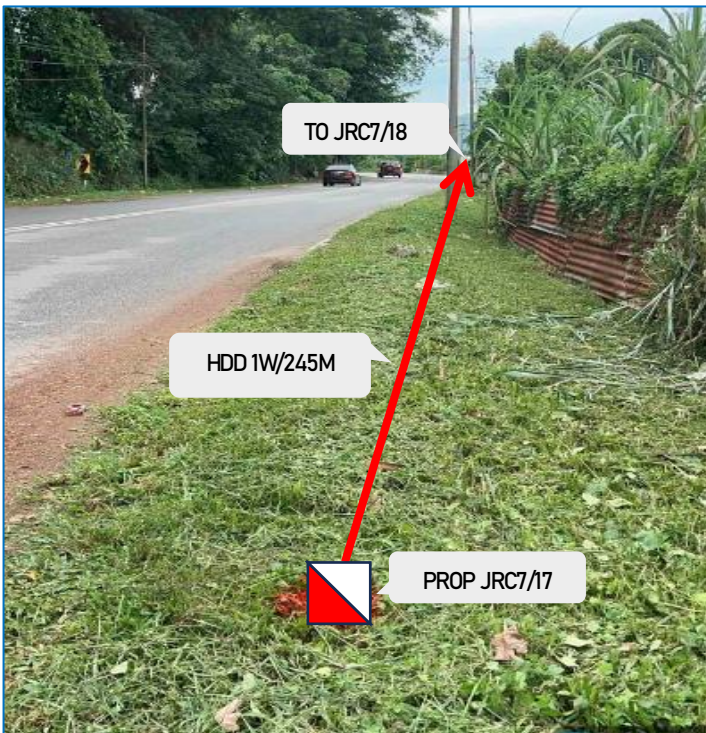
PROP JRC7/17 LOC AT JALAN AMPANG (ROADSIDE)
