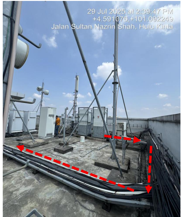
Picture 4 –CABLE WAY TRUNKING 100M
