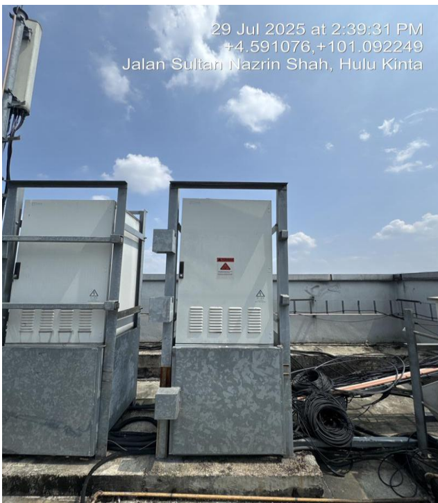
PICTURE 1 : CABINET UMOBILE
