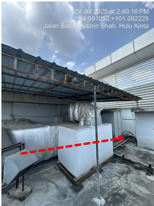
Picture 3 – CABLE WAY TRUNKING 100M
