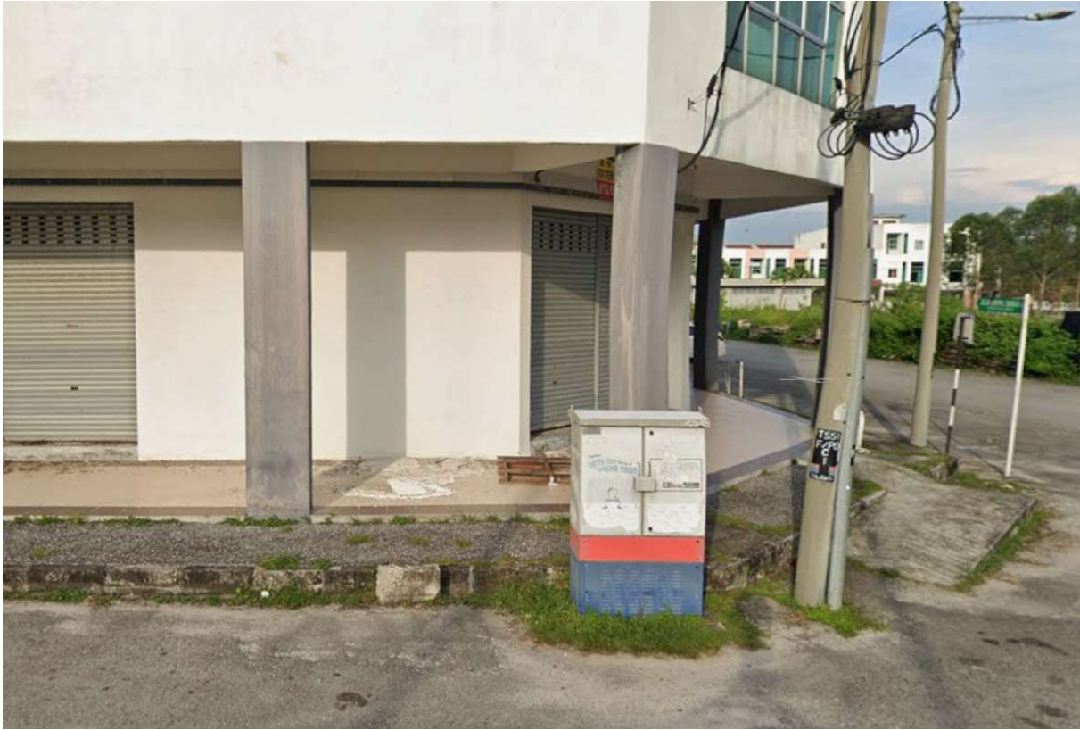
Gambar 3 : Feeder Pillar 400A Sedia Ada
