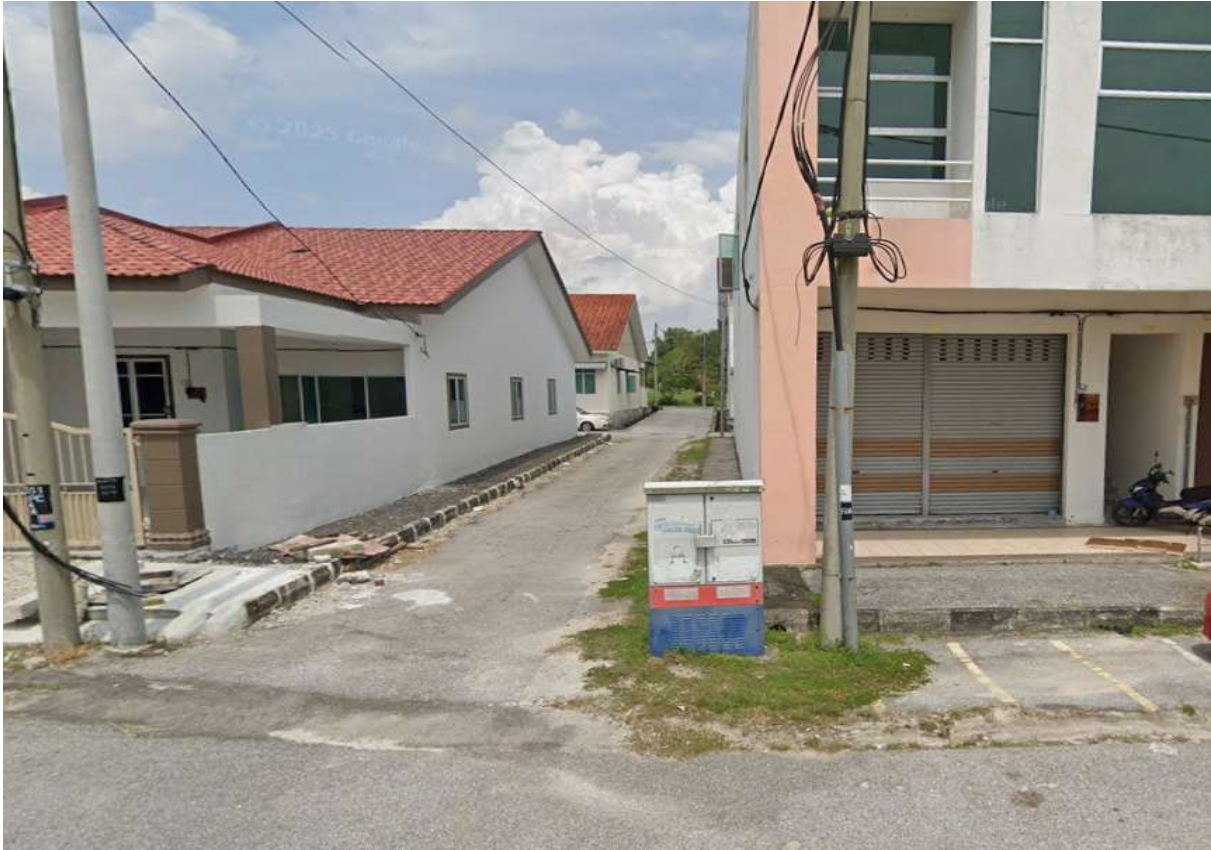
Gambar 1 : Feeder Pillar 400A Sedia Ada
