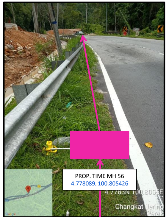
Proposed HDD 1 Way and Pulling Cable 144C from Prop. TIME MH56 to Prop. TIME MH57 at beside the highway
