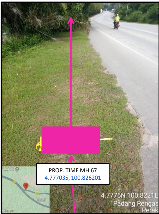
Proposed HDD 1 Way and Pulling Cable 144C from Prop. TIME MH67 to Prop. TIME MH68 at Jalan Abdul Shukor
