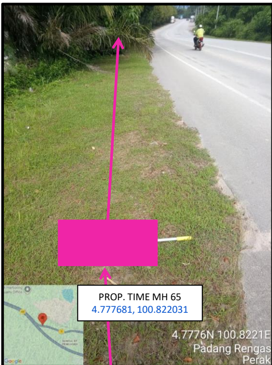
Proposed HDD 1 Way and Pulling Cable 144C from Prop. TIME MH65 to Prop. TIME MH66 at beside the highway
