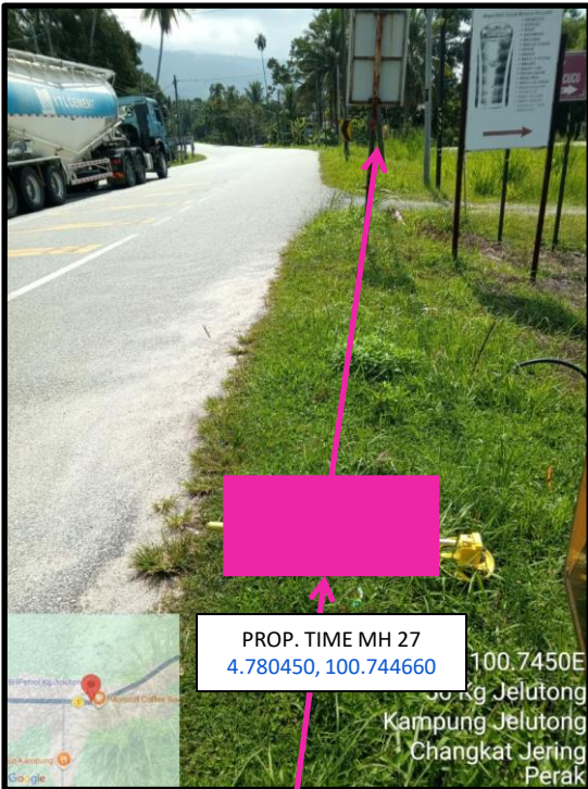
Proposed HDD 1 Way and Pulling Cable 144C from Prop. TIME MH27 to Prop. TIME MH28 at Jalan Enam Kaki
