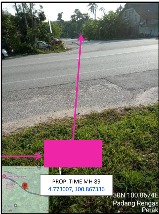
Proposed HDD 1 Way and Pulling Cable 144C from Prop. TIME MH89 to Prop. TIME MH90 at Padang Rengas
