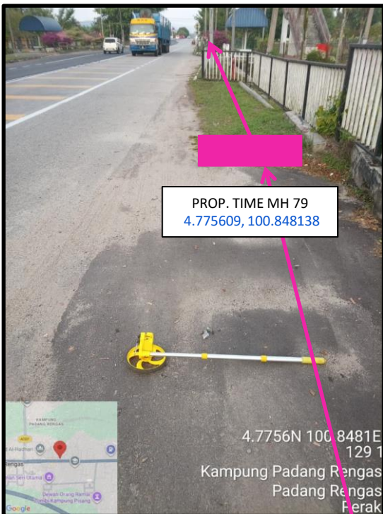
Proposed HDD 1 Way and Pulling Cable 144C from Prop. TIME MH79 to Prop. TIME MH80 at Kampung Padang Rengas
