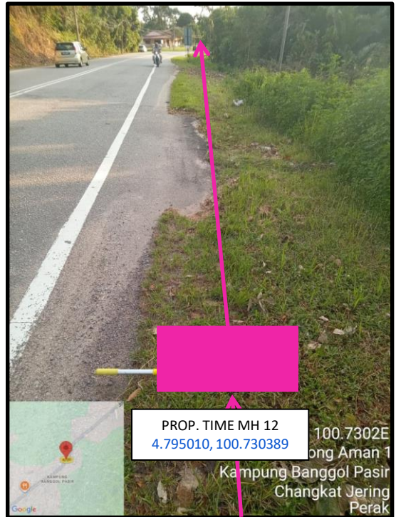
Proposed HDD 1 Way and Pulling Cable 144C from Prop. TIME MH12 to Prop. TIME MH13 at Jalan Air Kuning
