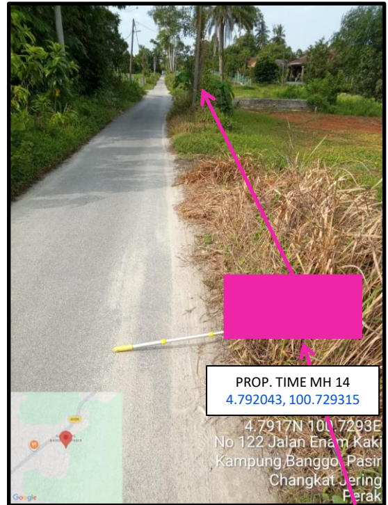
Proposed HDD 1 Way and Pulling Cable 144C from Prop. TIME MH14 to Prop. TIME MH15 at Jalan Enam Kaki
