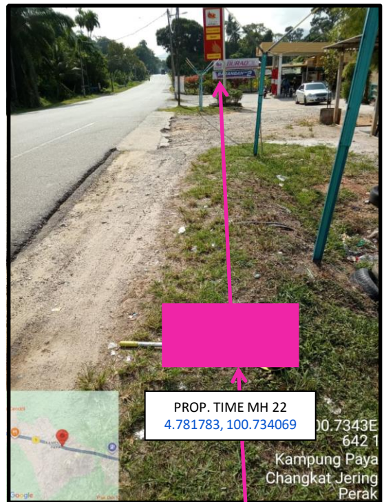
Proposed HDD 1 Way and Pulling Cable 144C from Prop. TIME MH22 to Prop. TIME MH23 at Kampung Paya
