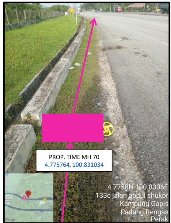
Proposed HDD 1 Way and Pulling Cable 144C from Prop. TIME MH70 to Prop. TIME MH71 at Jalan Abdul Shukor
