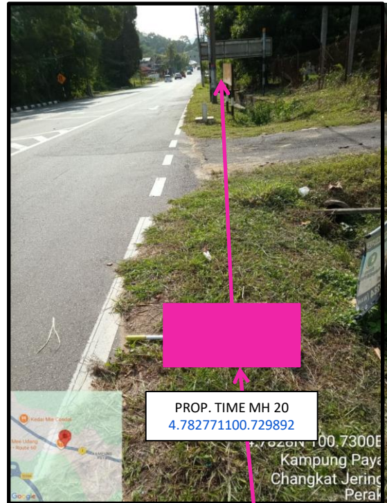
Proposed HDD 1 Way and Pulling Cable 144C from Prop. TIME MH20 to Prop. TIME MH21 at Kampung Paya
