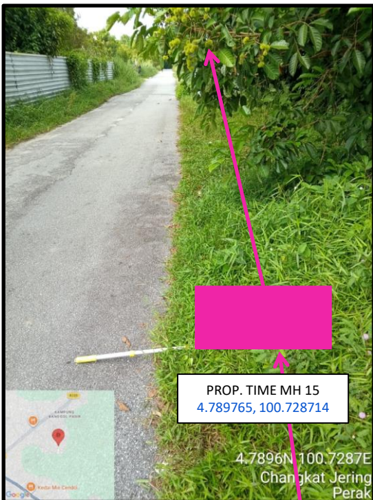
Proposed HDD 1 Way and Pulling Cable 144C from Prop. TIME MH15 to Prop. TIME MH16 at Jalan Enam Kaki
