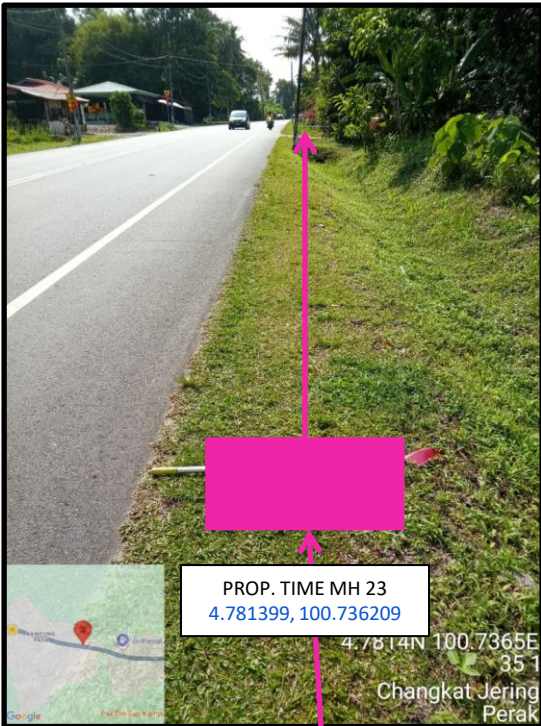
Proposed HDD 1 Way and Pulling Cable 144C from Prop. TIME MH23 to Prop. TIME MH24 at Kampung Paya
