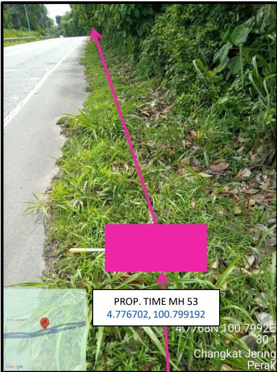
Proposed HDD 1 Way and Pulling Cable 144C from Prop. TIME MH53 to Prop. TIME MH54 at beside the highway
