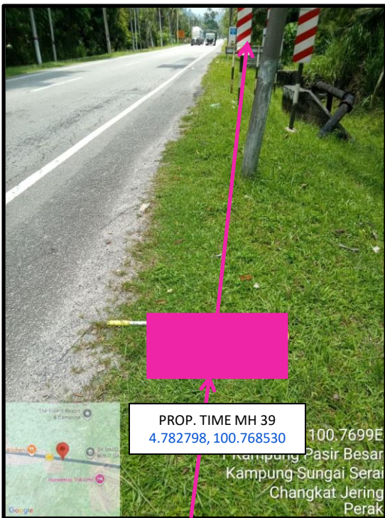
Proposed HDD 1 Way and Pulling Cable 144C from Prop. TIME MH39 to Prop. TIME MH40 at Kampung Pasir Besar
