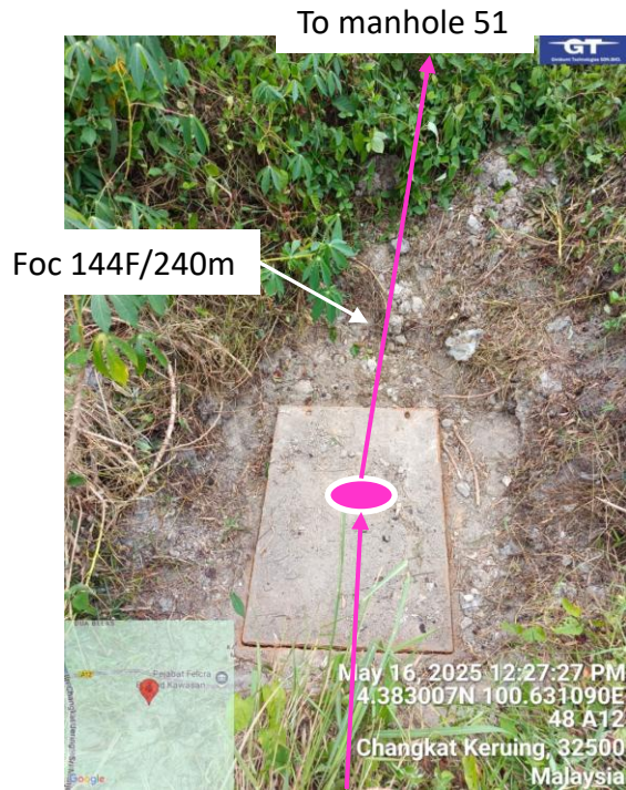
Manhole 50 Way ok Mh 51 to Mh 50, Manhole need to raise up
