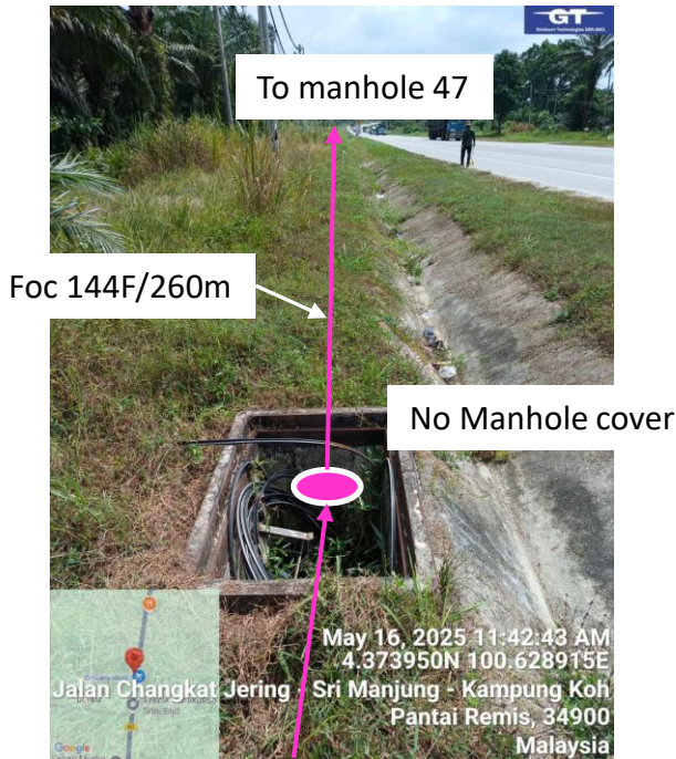
Manhole 46 Way blockage 1.5m cw dummy subduct Mh 46 to Mh 47 (30m(1.5) & Manhole need to raise up
