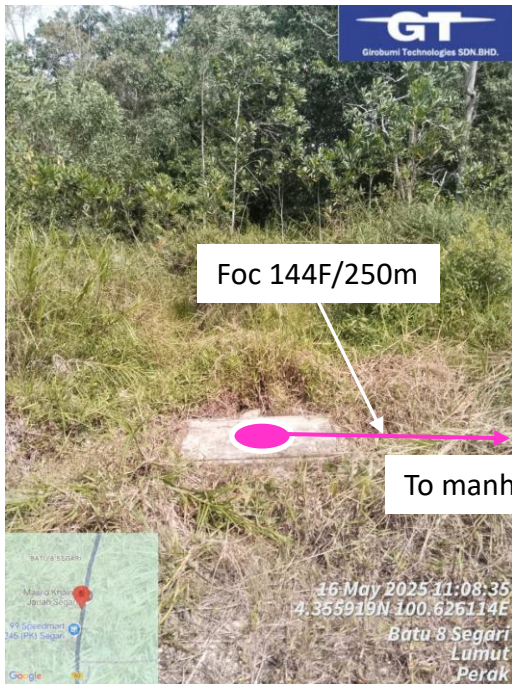
Manhole 38 Way rosak Mh 38 ke MH 39 (1m sangkut) Way rosak Mh 39 ke Mh 38 (1 subduct)
