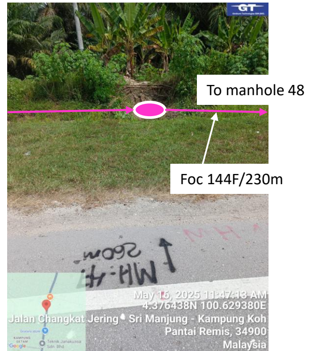
Manhole 47 Way blockage 1.5m cw dummy subduct Mh 48 to Mh 47 block 190m(1.5m) & Manhole need to raise up
