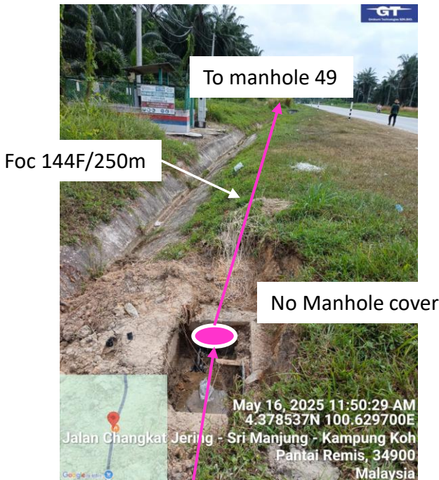
Manhole 48 Way blockage cw dummy subduct Mh 49 to Mh 48, river crossing & Manhole need to raise up. Prop New HDD Mh 48 to Mh 49.
