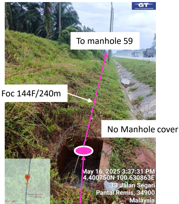
Manhole 58 Way ok Mh 58 to Mh 59 Manhole need to raise up
