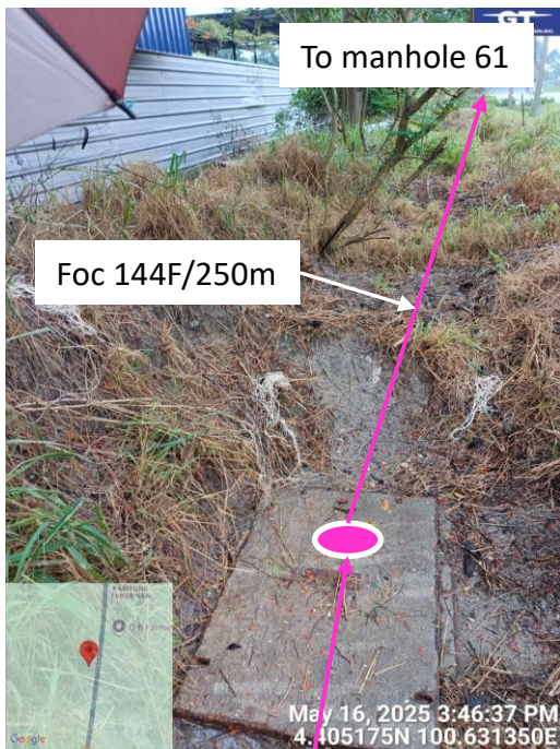
Manhole 60 Way ok Mh 60 to Mh 61 Manhole need to raise up
