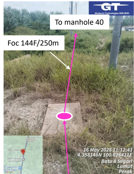
Manhole 39 (210m(1.17m) Blokage Mh 40 to Mh 39)
