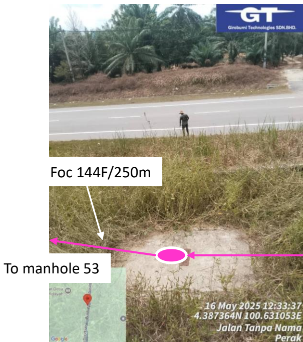
Manhole 52 Way problem, pipe broken & dummy subduct to Mh 52 to Mh 53. Prop New HDD Mh 52 to Mh 53
