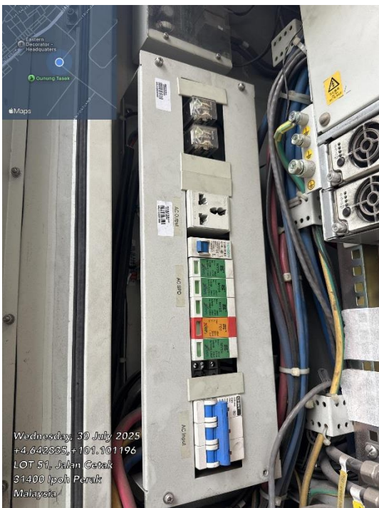
Picture 3 – DC POWER SOURCE
