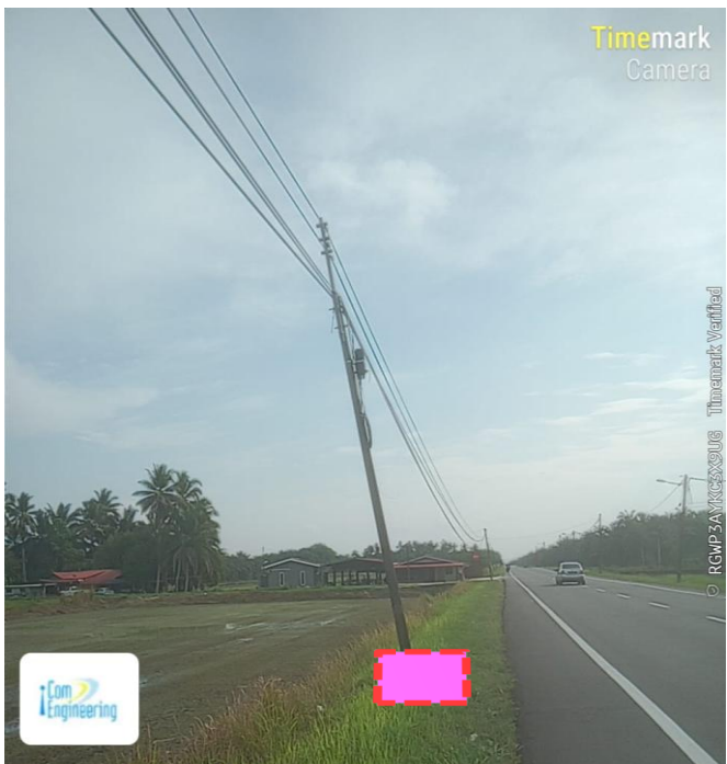
Prop New TIME MH 43 (Jalan Labu Kubong) (4.116819, 101.074310)
