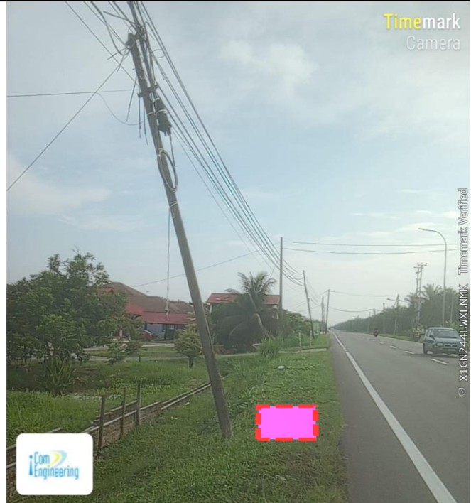
Prop New TIME MH 41 (Jalan Labu Kubong) (4.119377, 101.077848)
