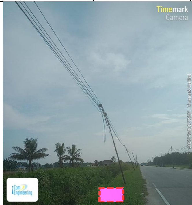
Prop New TIME MH 49 (Jalan Labu Kubong) (4.109330, 101.063632)
