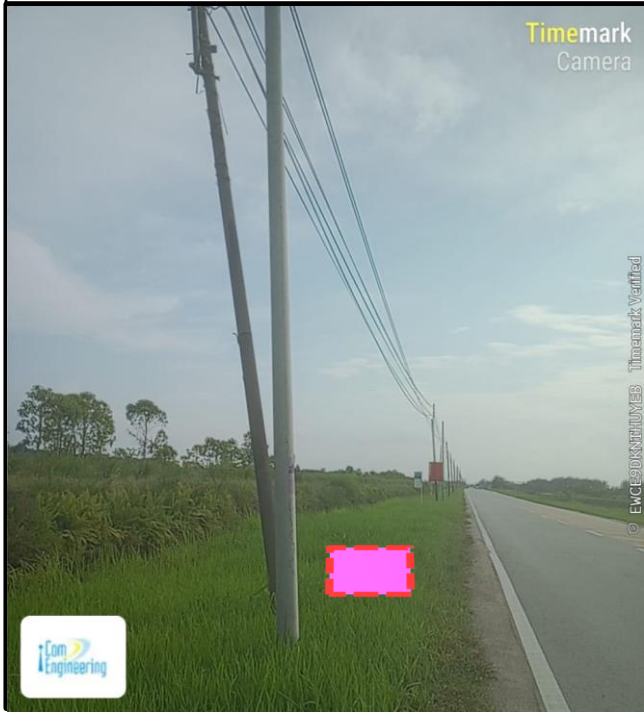
Prop New TIME MH 52 (Jalan Labu Kubong) (4.105456, 101.058309)
