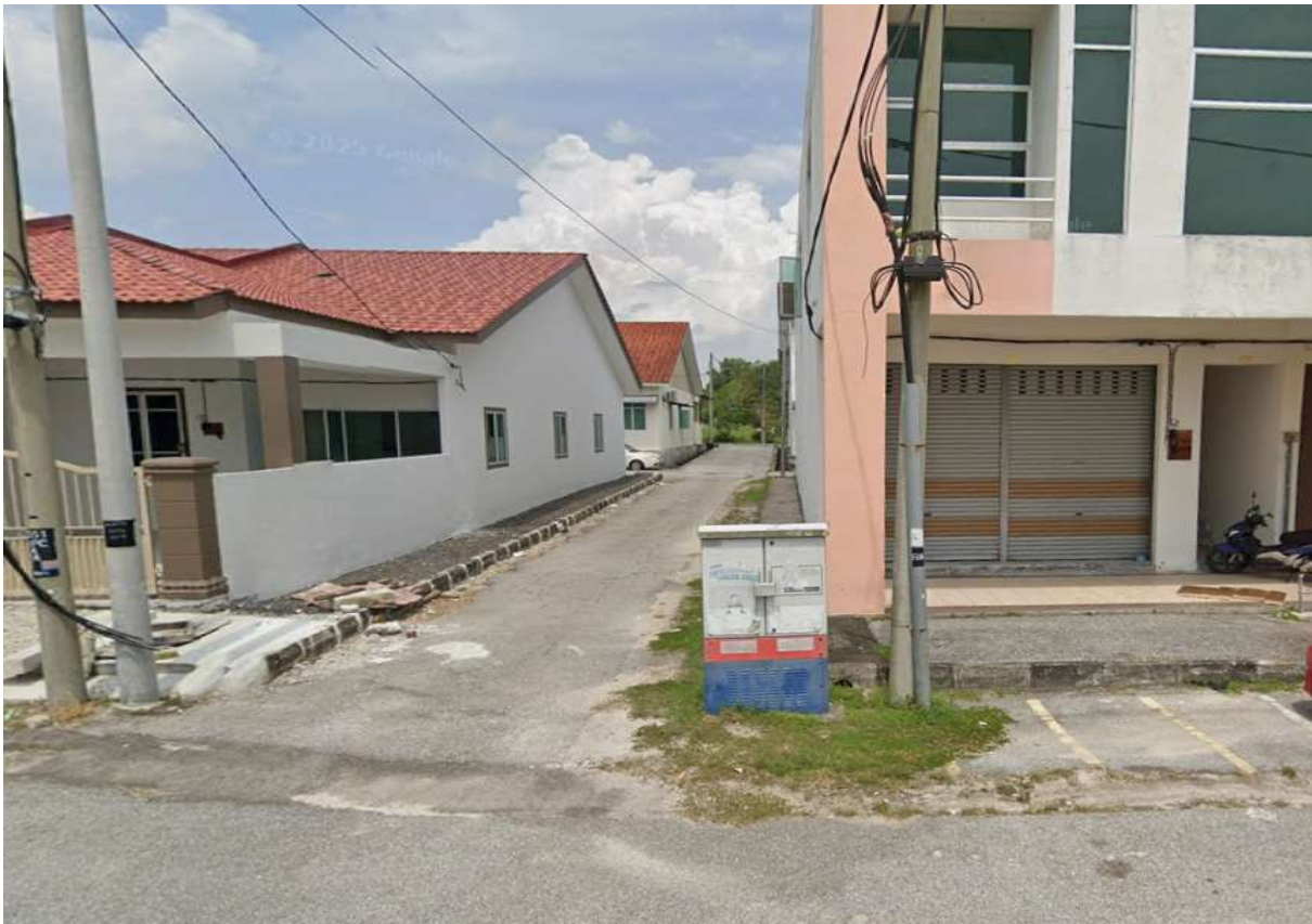
Gambar 1 : Feeder Pillar 400A Sedia Ada
