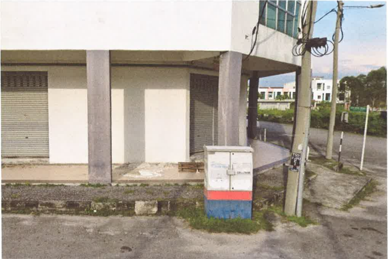
Gambar 3 : Feeder Pillar 400A Sedia Ada
