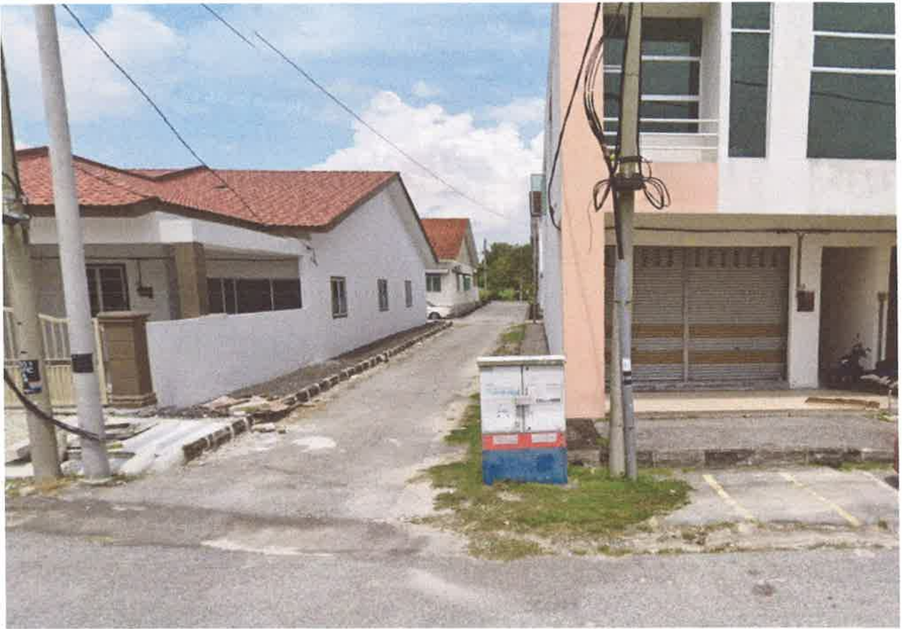
Gambar 1 : Feeder Pillar 400A Sedia Ada
