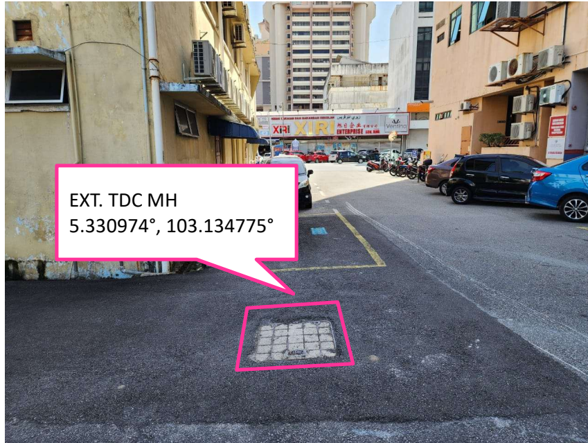
Existing TDC Manhole (Pro. Joint MH)
