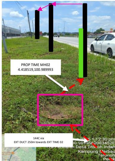
Existing TIME MH02 and prop 144C Cable pulling via pole to EXT TIME MH03 at Ipoh – Lumut Highway (JKR)
