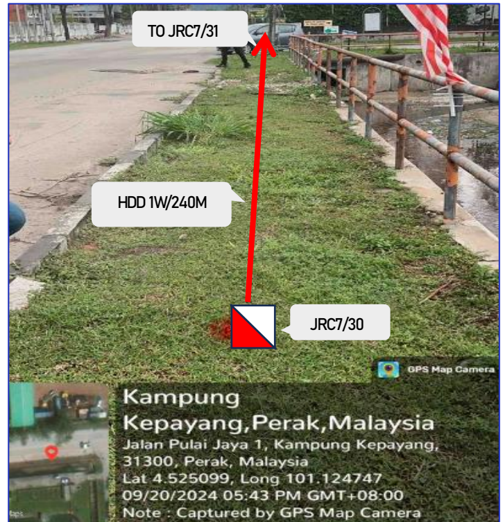
PROP JRC7/30 AT JALAN PULAI JAYA 1 (ROADSIDE)
