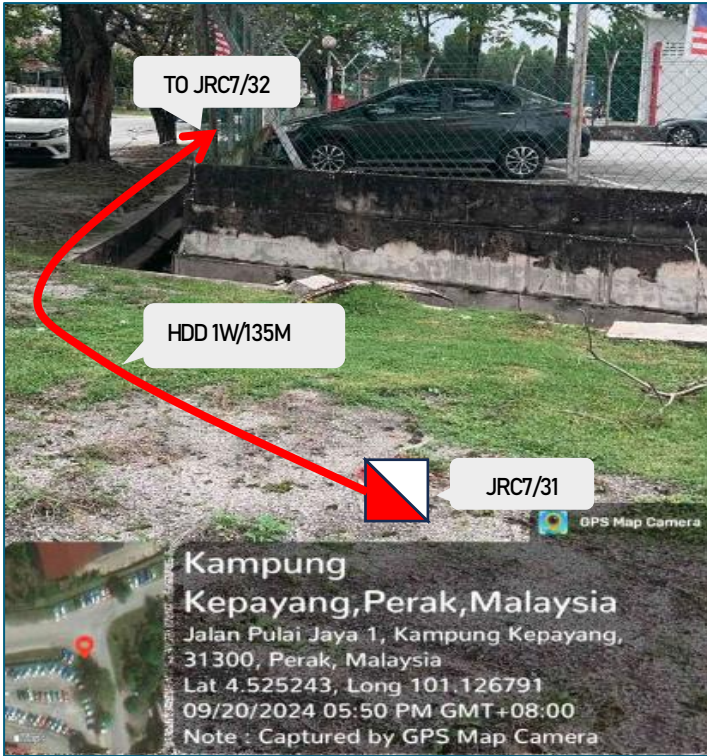
PROP JRC7/31 AT JALAN PULAI JAYA 2 (ROADSIDE)
