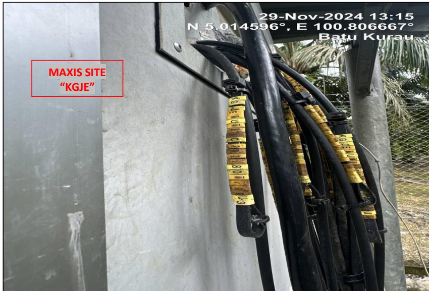
LOCATION AT MAXIS SITE KGJE
