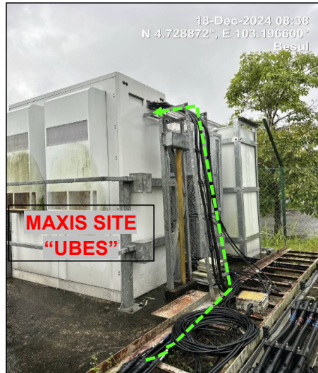
LOCATION AT MAXIS SITE "UBES"
