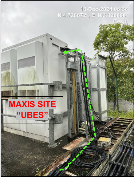
LOCATION AT MAXIS SITE"UBES"
