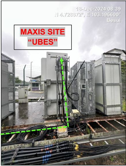
LOCATION AT MAXIS SITE "UBES"
