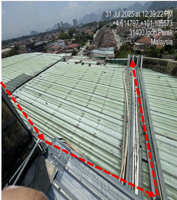
Picture 3 – CABLE WAY TRUNKING
