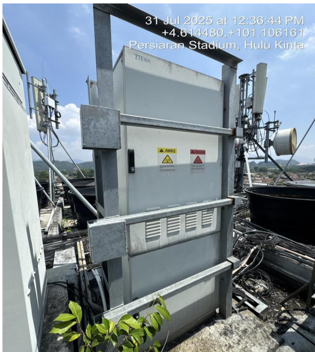
PICTURE 1 : CABINET UMOBILE
