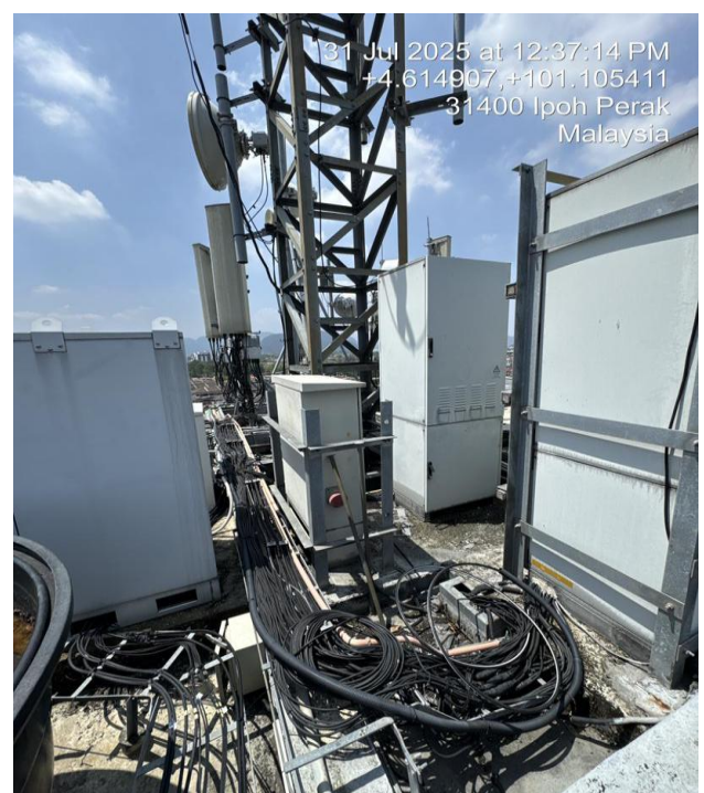
Picture 2 – CABLE WAY TRUNKING
