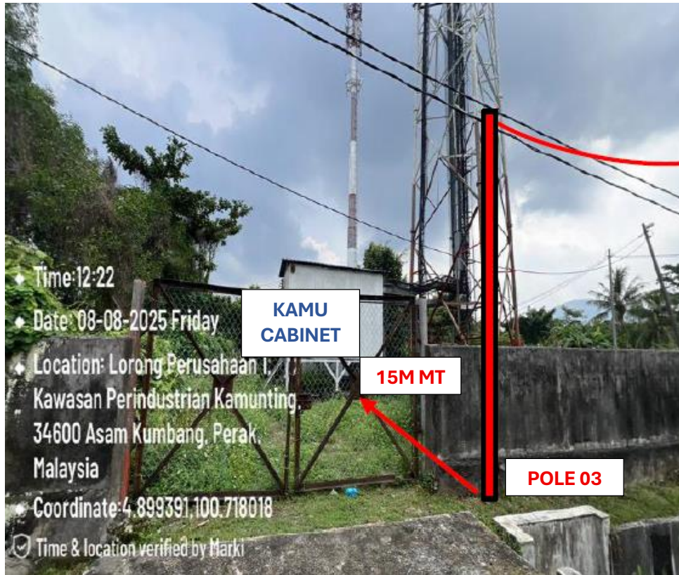
PICTURE 5 : POLE 03 TO KAMU CABINET
