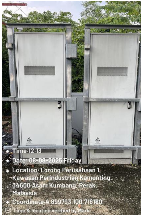
PICTURE 1 : KIKT CABINET
