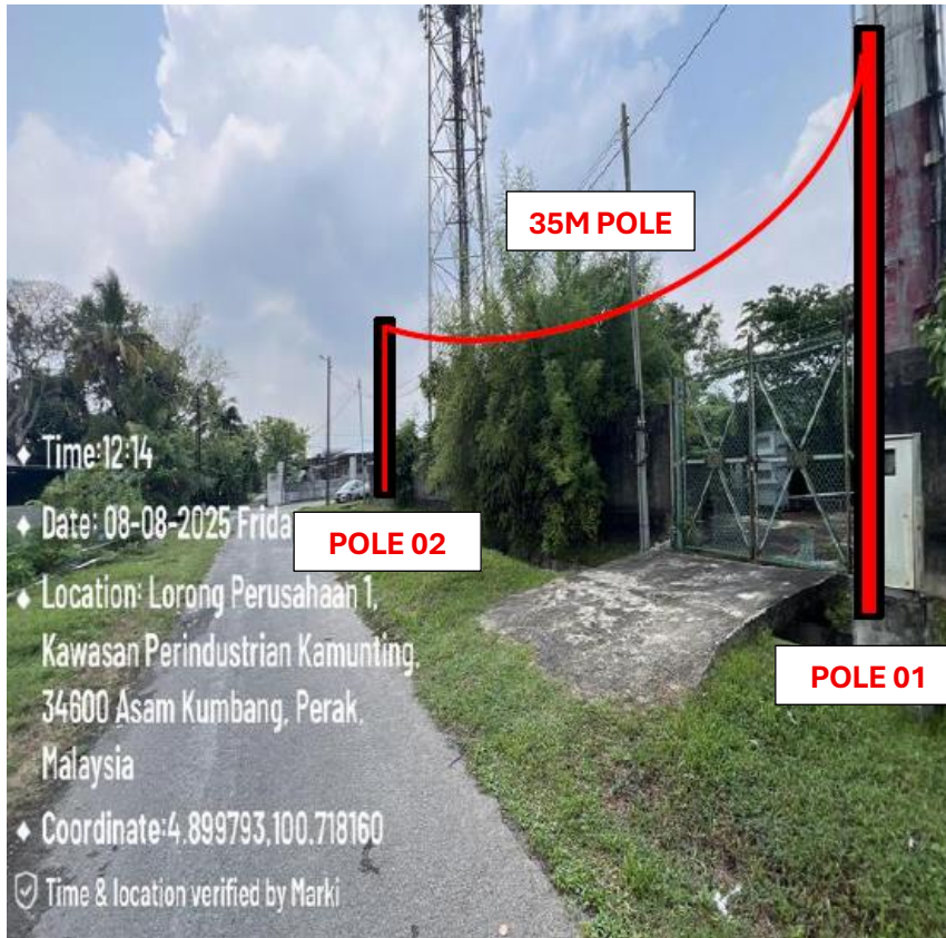
PICTURE 3 : POLE 01 TO POLE 02
