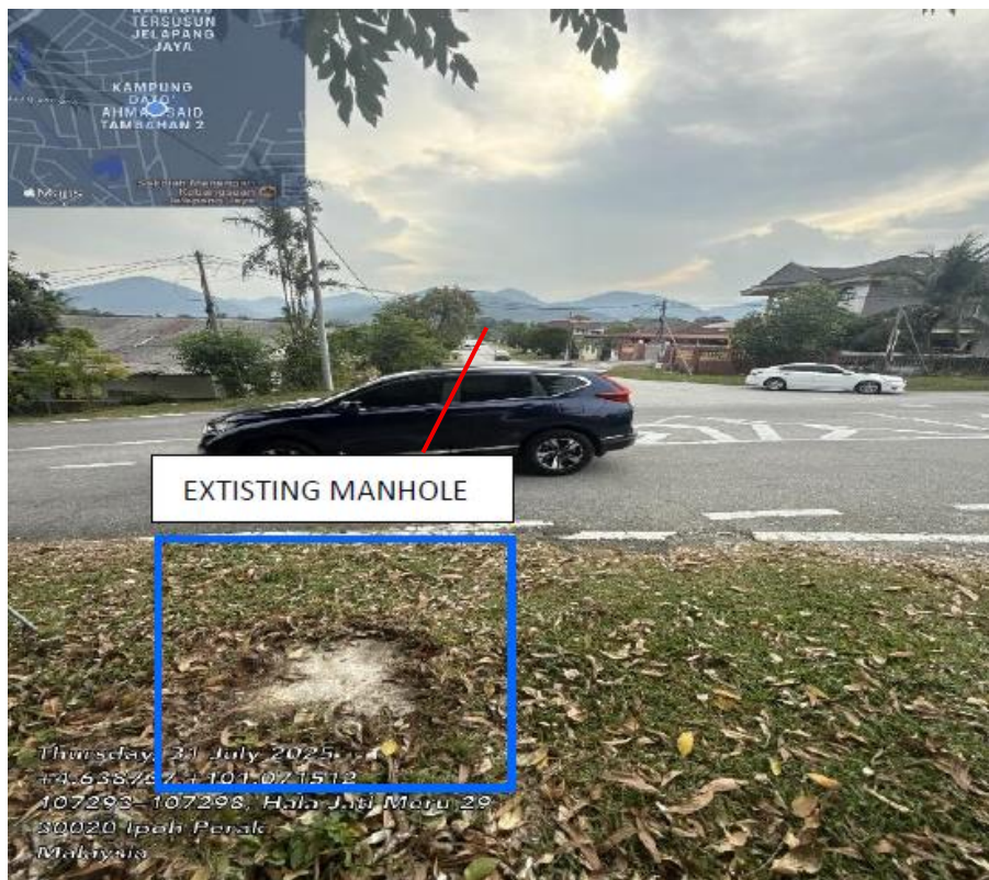
PICTURE 1 : EXISTING MAXIS MH
